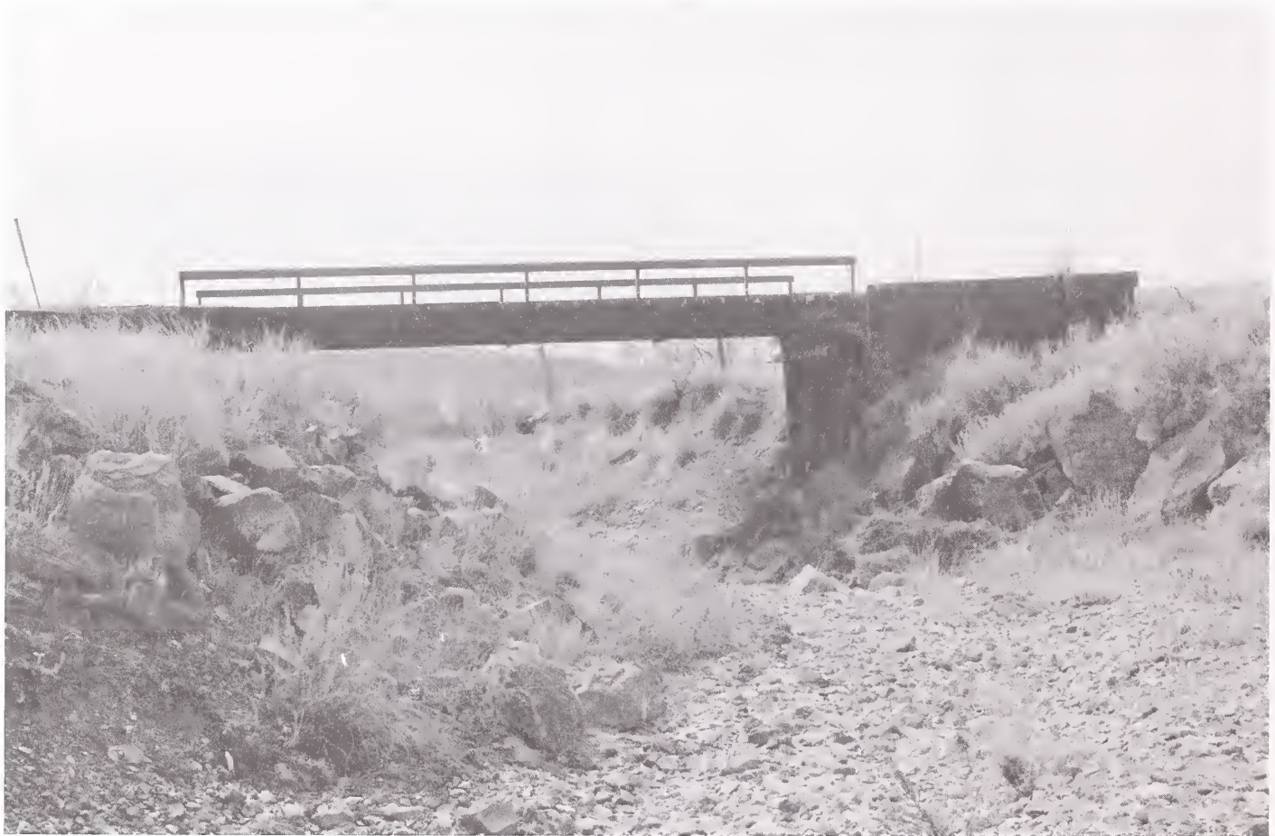
Constructed in 1901, the Locate Creek Bridge is the oldest known steel stringer bridge in the state.
